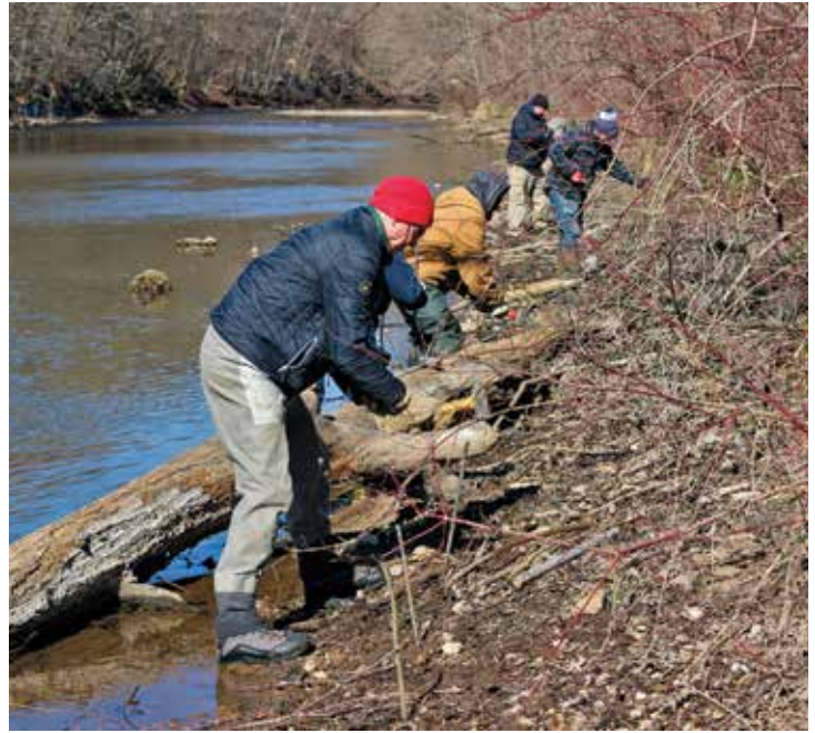
Volunteers from Aqua and the Montgomery County Conservation District, the Perkiomen Valley Trout Unlimited, and Montgomery County Master Watershed Stewards installed 200 live stake plantings to stabilize the newly exposed stream banks.
